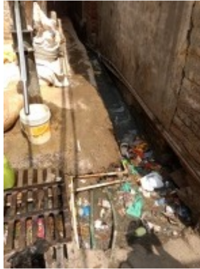
(b) Garbage and plastic bags clog drains. Blockage in one section can lead to overflows throughout the settlement.
