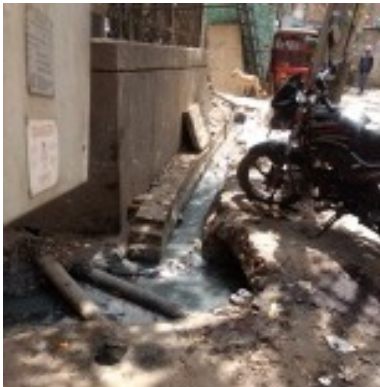
Internal drain from basti connecting to the main drain in Site C
