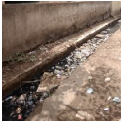
Main drainage clogged with garbage in Site D
