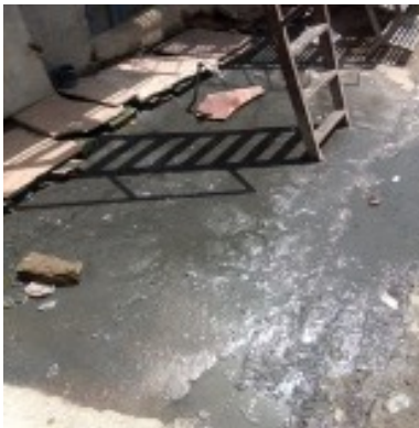
Overflowing drains in Site A
